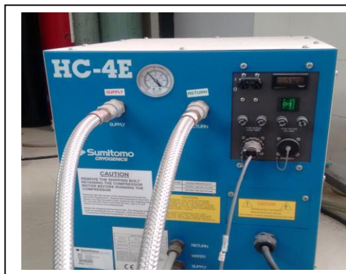
(h): Helium compressor
